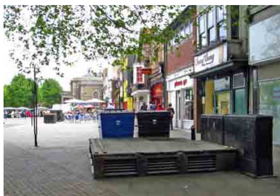
Existing substation in the south-west corner of the site
