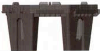
Large void space between columns
